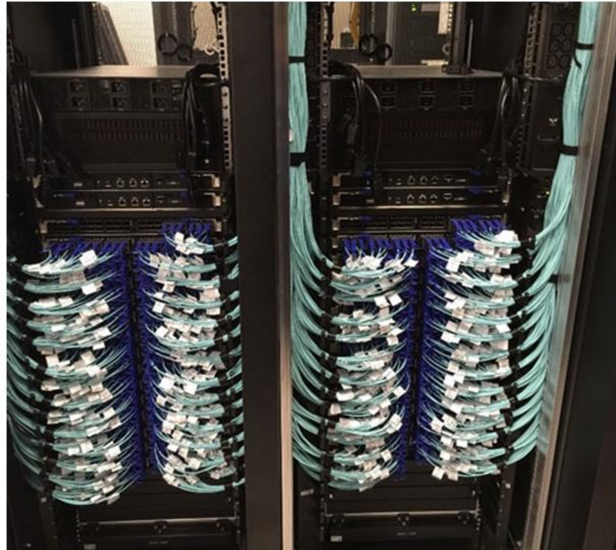
Example of proper cable management
